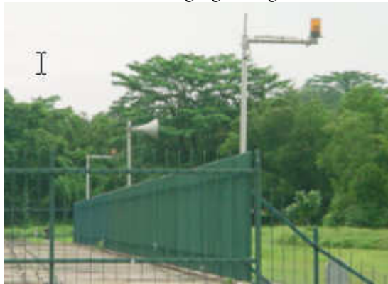
Photo 7: Beacons and warning signs
